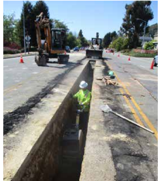
We replaced over 10,000 linear feet of water main pipelines on Soquel Drive.
