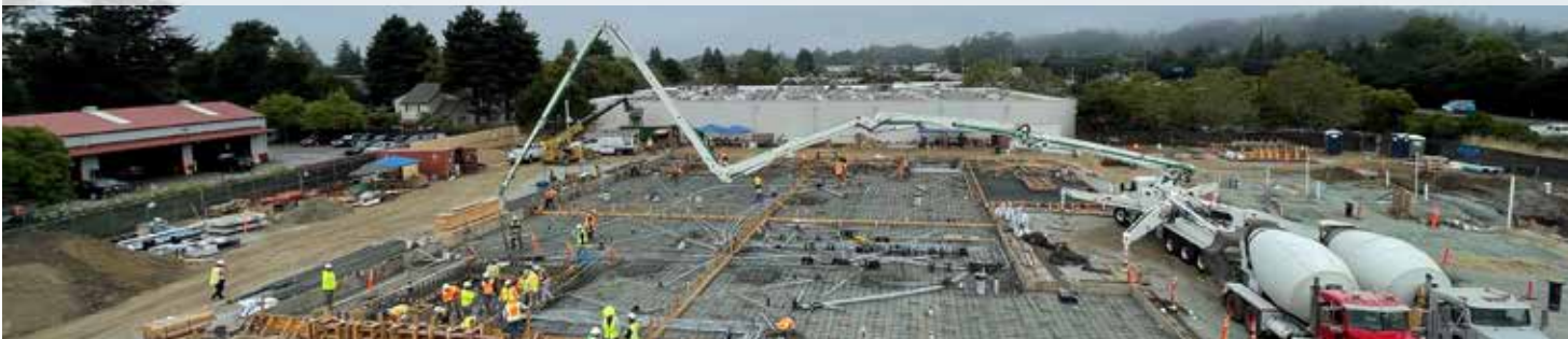
Water Purification Center being constructed at the corner of Chanticleer Ave. and Soquel Ave.
